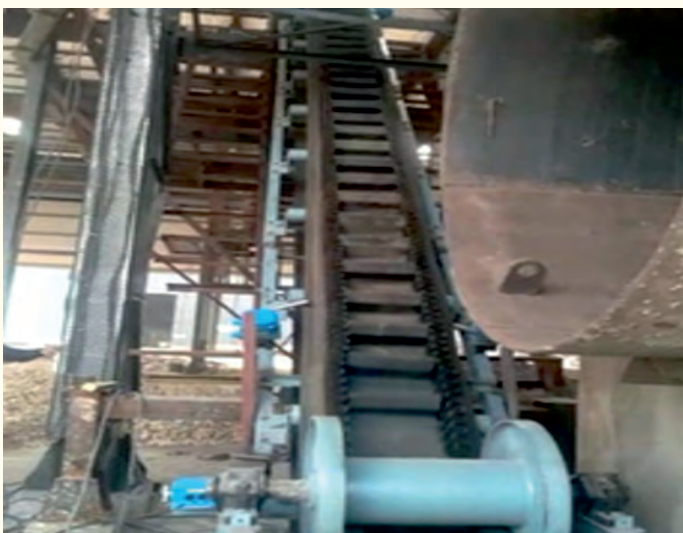
High Angle Conveyor
